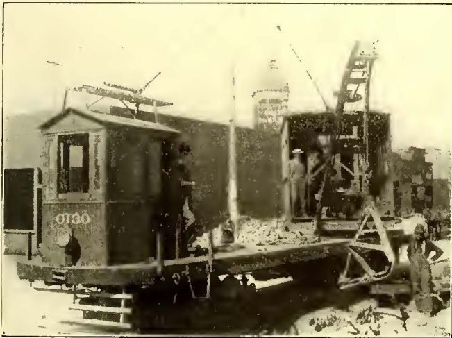
San Francisco Street Railways—Reconstruction of Hayes Street, Showing Method of Pulling Yokes with Crane Car
