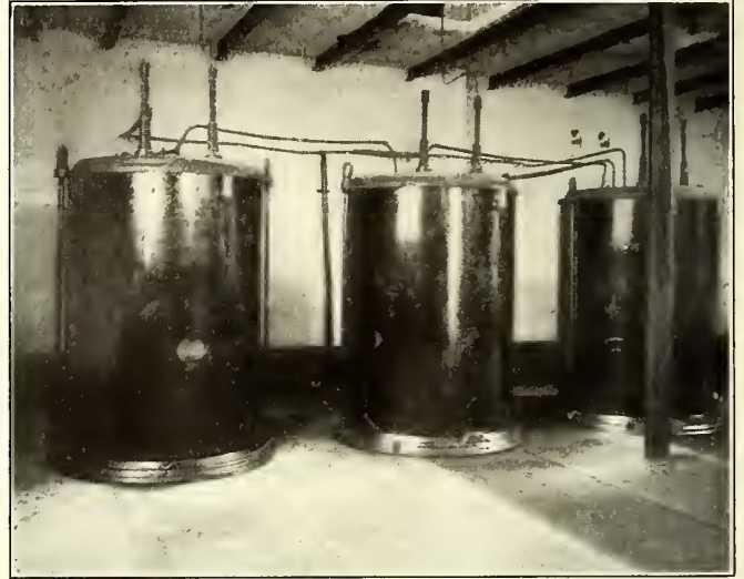
San Anselmo Substation—Oil-Cooled, Shell Type Transformers
