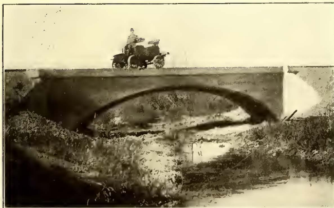
Fig. 7.—Bridge Reconstruction on Columbus & Lake Michigan Railway—Bridge 401, 35-ft. Span on a 30-deg. Skew
