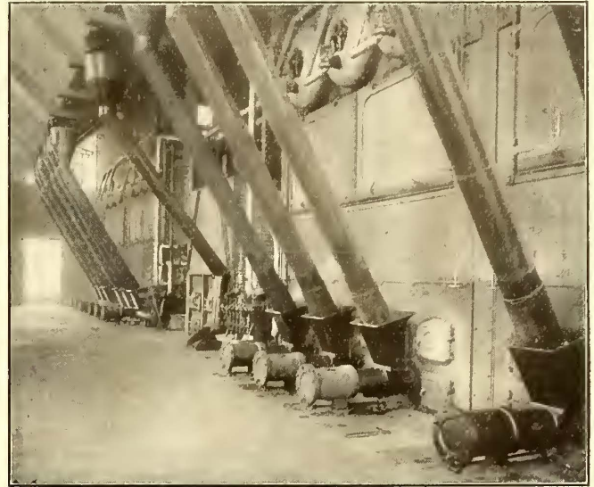
St. Clair Tunnel Electrification—Boiler Room in Power Station at Port Huron
