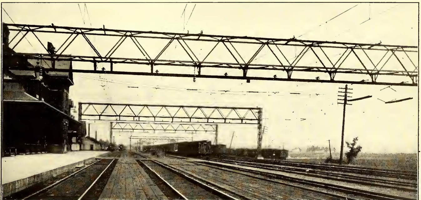
St. Clair Tunnel Electrification—Overhead Construction at Port Huron Station Spanning Eight Tracks
