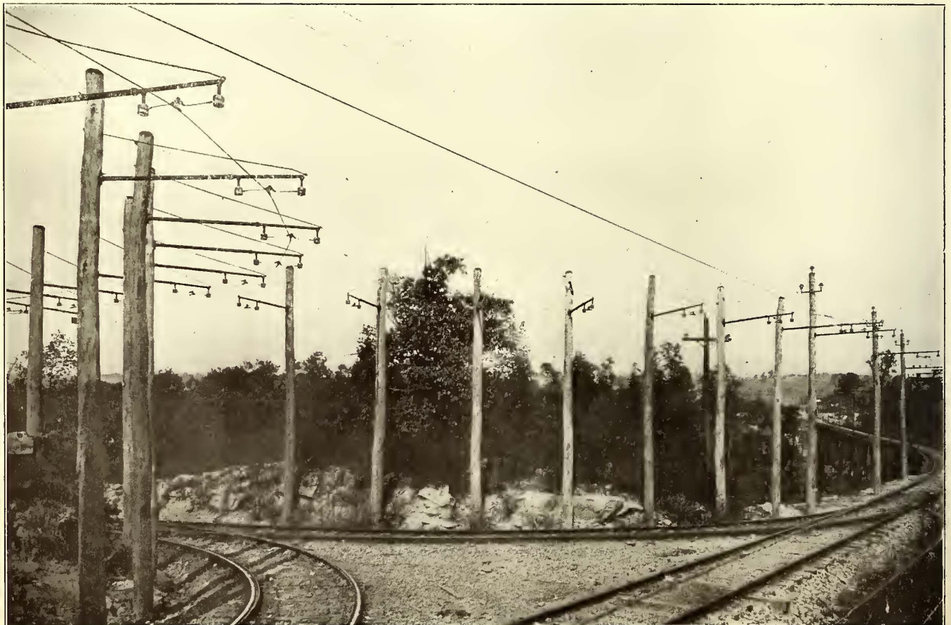
Pittsburg 1200-Volt Line—Ellwood City Y
