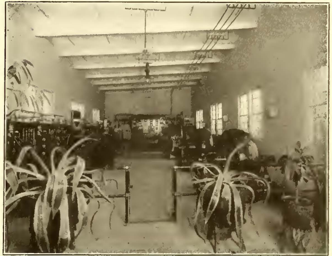
Binghamton Railway—Interior of Sub-Station No. 1 at Endicott, N. Y.
