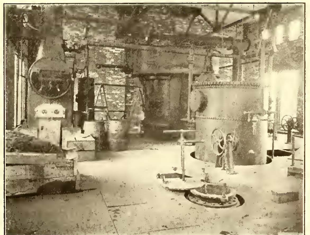
Producer Room of Boston Elevated Railway Somerville Gas Engine Power Station
