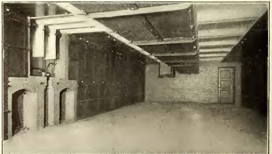
Baltimore Switchboard—View in Basement
