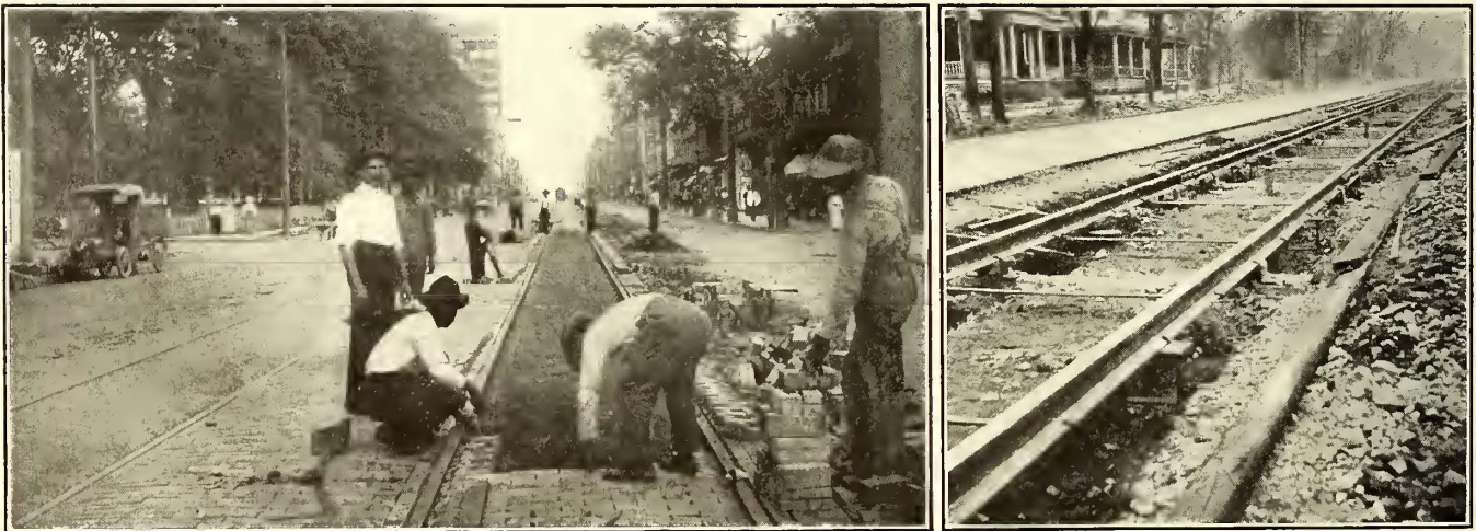
T-Rail in Charlotte, N. C.—Laying Brick Pavement Between Rails and Track Prepared for Concrete Base
