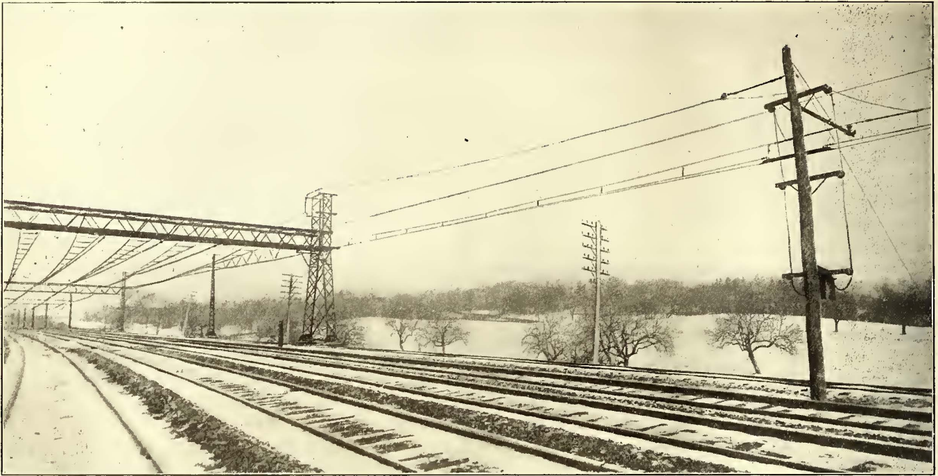
New Canaan Electrification—View at Junction with the Main Line, Illustrating the Difference in Overhead Construction Between Heavy and Light A.C. Operation
