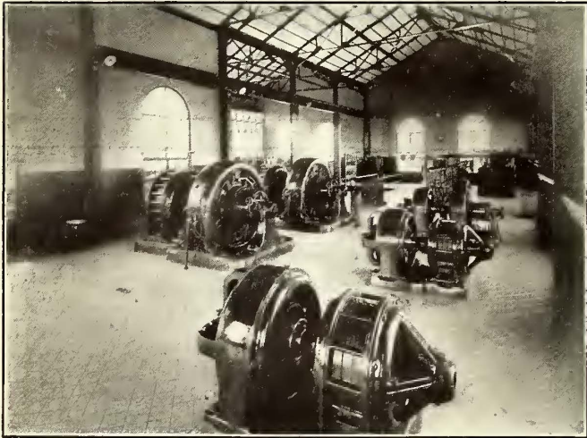
Mexico City Tramways—Churubusco Substation, Illustrating the Use of Motor-Generator Sets
