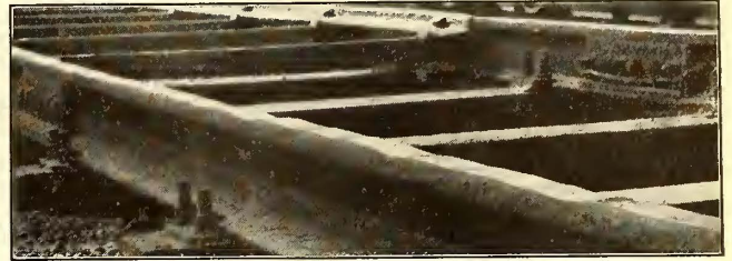
Fig. 3—Badly Corrugated Rail on Triangular Curve of Berlin Elevated Railway
