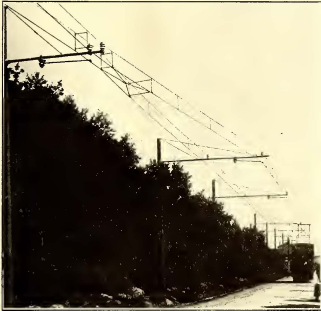
Lyons Single-Phase Tramways—Rectangular Separators at a Siding
