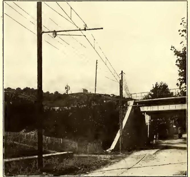
Lyons Single-Phase Tramways—Plain Catenary Brackets on Channel and Tubular Poles
