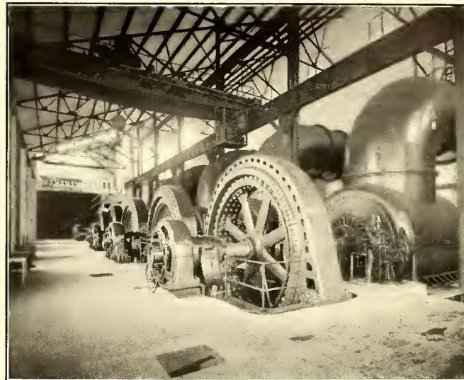
Washington Water Power Company—Interior of Post Falls Power Station
