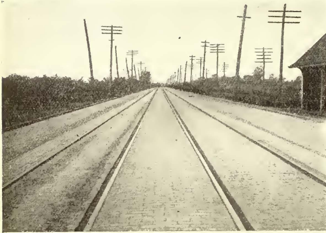
Way Matters—Track in Utica, N. Y., Laid in 1908, with 100-lb. Open-Hearth T-Rail, Steel Ties, Concrete Foundation, Clark Joints
