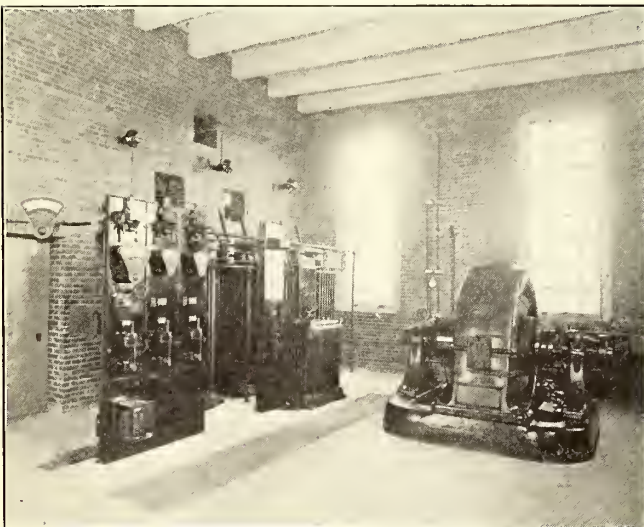
Maine Electric Railways—Substation at Day's Corner
