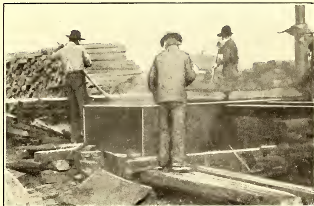
Treating Ties in Metal Tank
