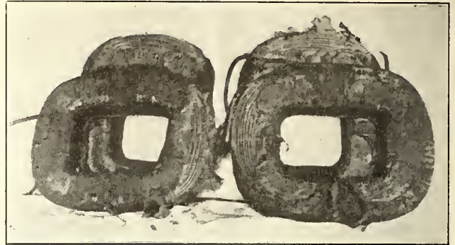
Field Coils Ruined Through Neglect in Cutting Out a Damaged Motor
