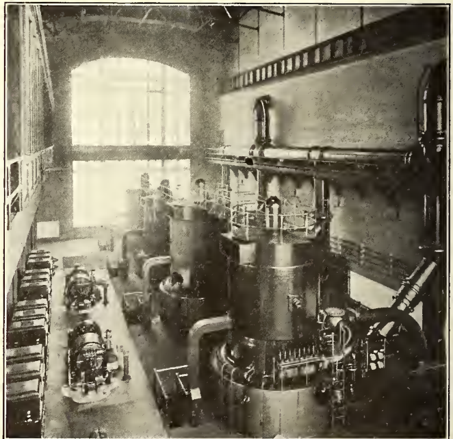
Hudson & Manhattan Railroad Power Station—Generator Room, Looking Toward Boiler Room
