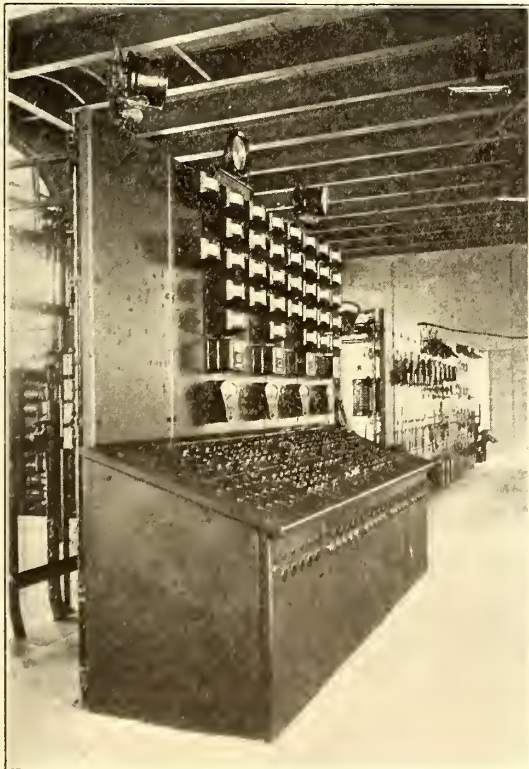
Hudson & Manhattan Railroad Power Station—Remote Control Panel
