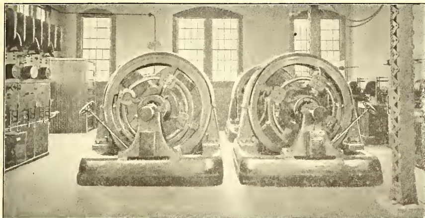
Change to 1200 Volts on W., B. & A.—Interior of Baltimore Substation, Showing the Rotary Converters Arranged in Pairs for Supplying Current at 1200 Volts
