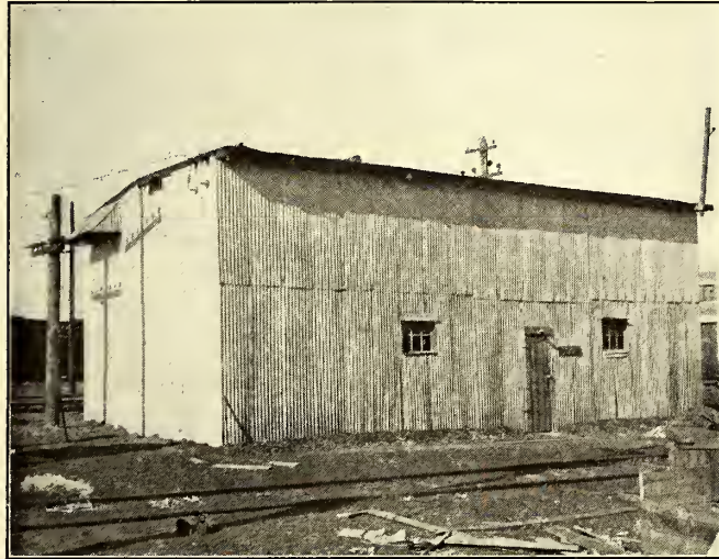
Change to 1200 Volts on W., B. & A.—Exterior View of the Temporary Substation at Naval Academy Junction, Showing Line Entrance
