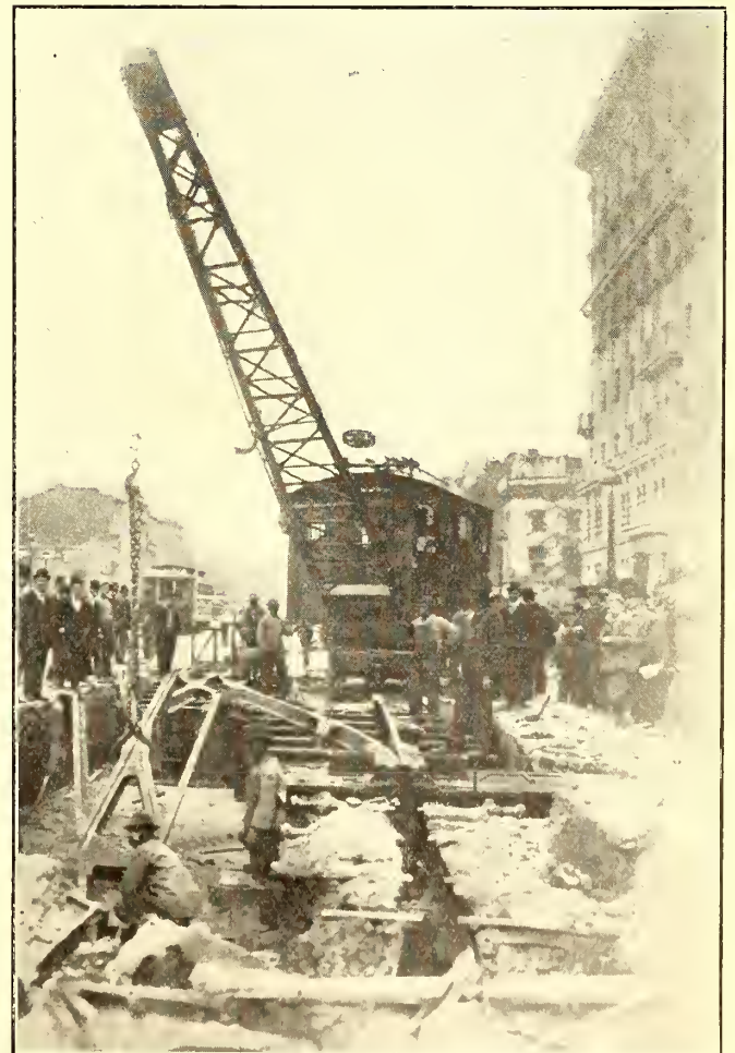
Conduit Reinforcement at Washington—Fig. 7—Electric Crane
