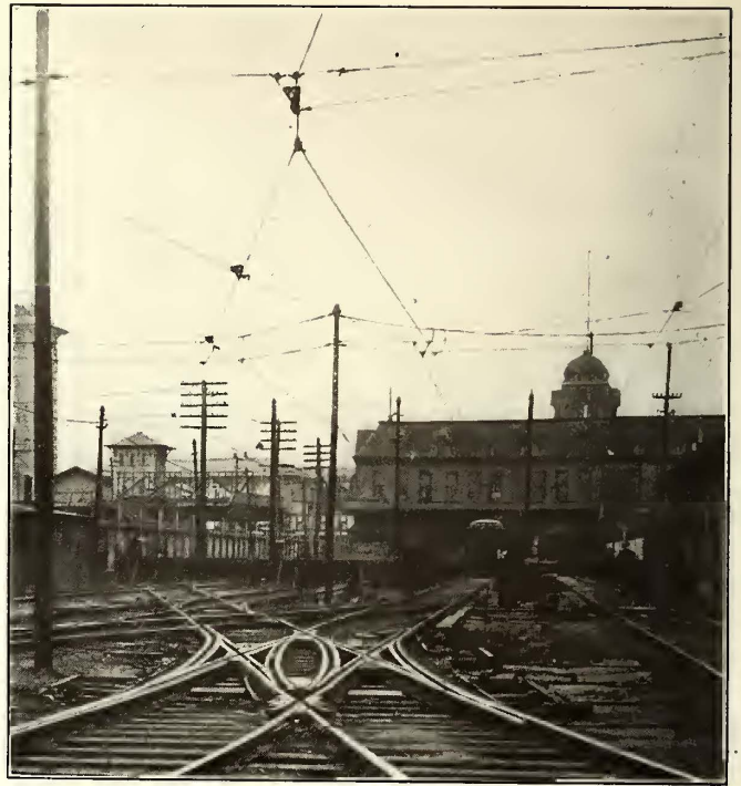
Brooklyn Line Department—Overhead Construction for Combined Switch and Cross-over at Coney Island
