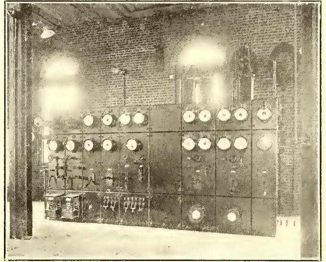
New York & North Shore Traction—Switchboard in Power Station
