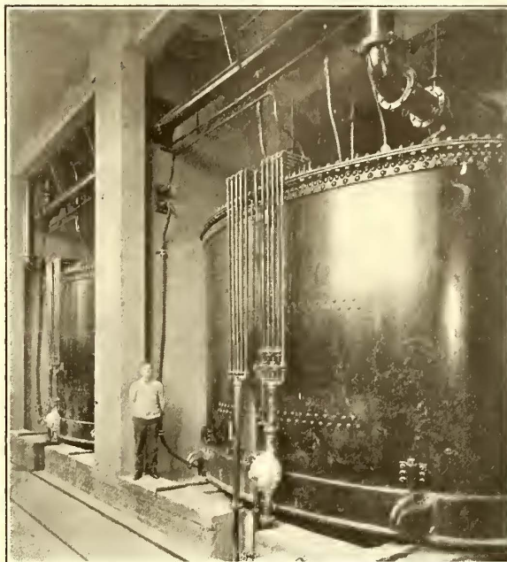
10,000-kva Transformer Installed in a Baltimore Substation for Power from McCall's Ferry
