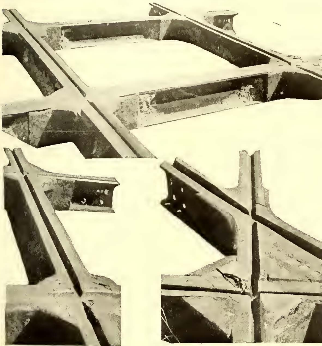
Views of Damaged Special Work Used as Object Lessons
