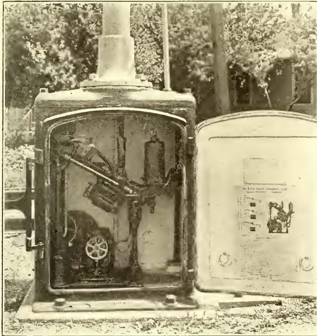
Illinois Traction Signals—Bottom Post Signal Mechanism
