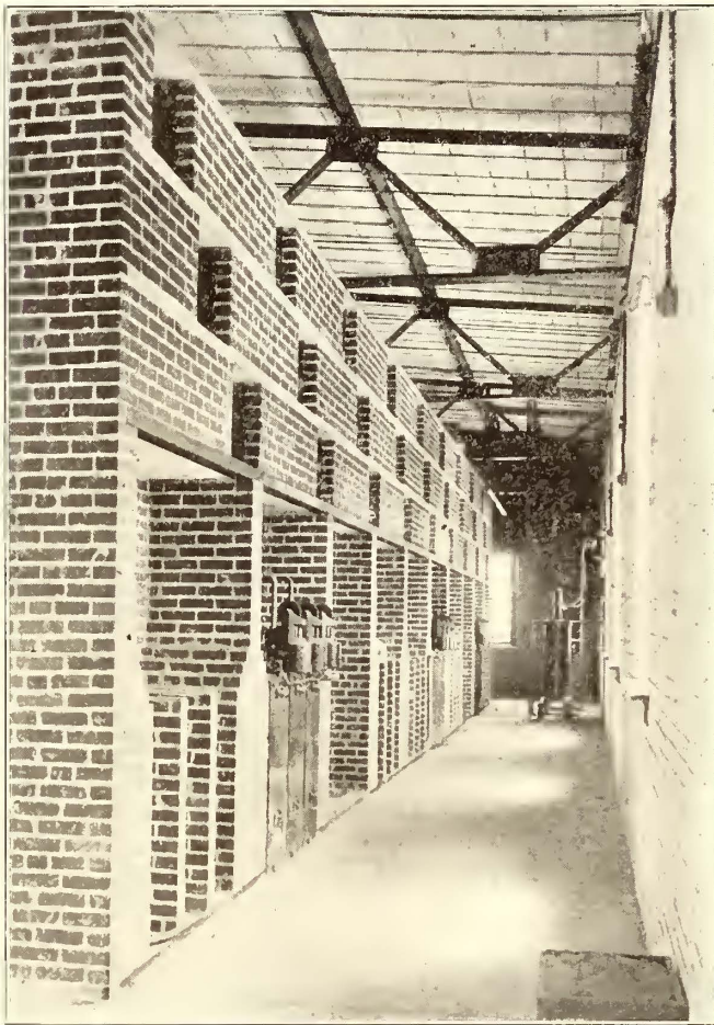
Illinois Traction Power Station—33,000-Volt Busbar Room
