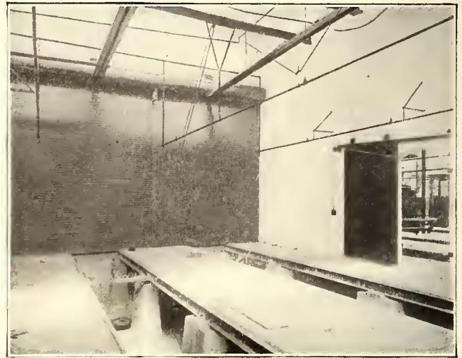
Bridgeport Carhouse—Steel Shutter for Isolating the Paint Shop from Rest of Maintenance Section
