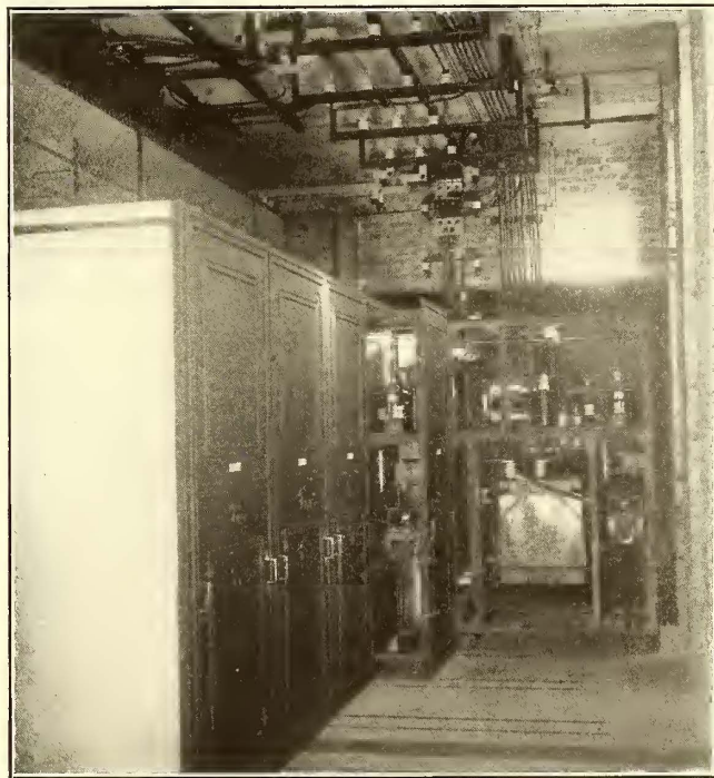
Schöneberg Subway—High-Tension Substation Apparatus in Castor-Mounted Cabinets for Quick Disconnection
