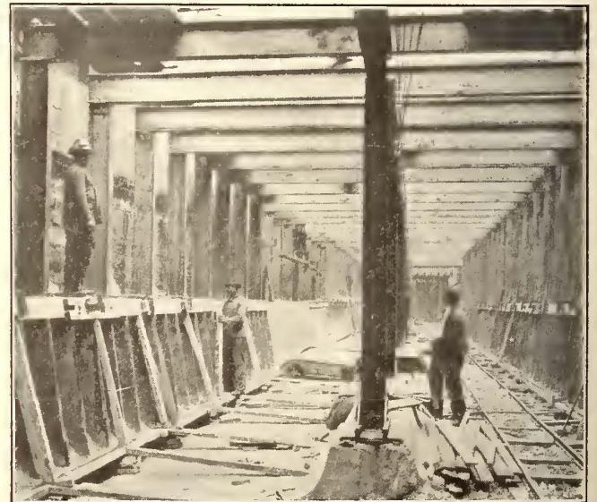
Schöneberg Subway—Erection of Structural Steel Work shaft is covered by grill work, which can be easily opened from below. The wide stairways at stations also are an appreciable factor in the ventilation of the subway. However, the most effective means for introducing fresh air en route is presented at the Stadtpark station, where the line passes through what is practically an open cut for 70 m (230 ft.).
