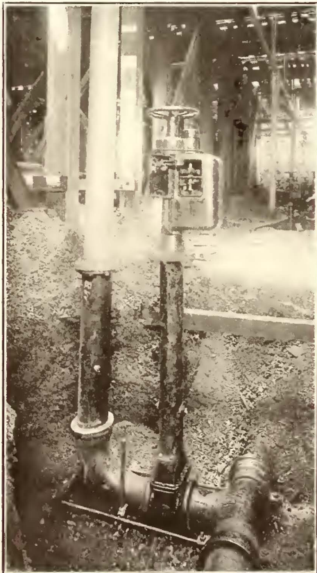
Manhattan Elevated Sprinklers—Motor-Operated Hydrant Valve
