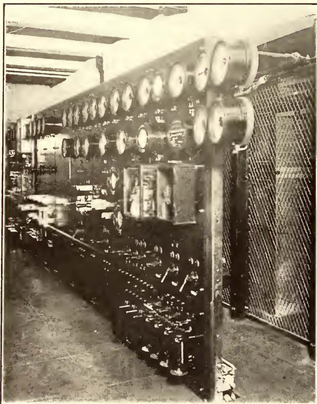
Hoosac Tunnel Power Station—Operating Switch Board
