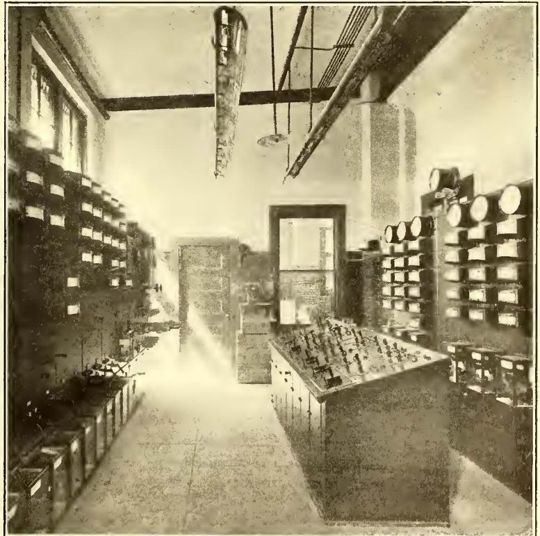
Jordan Power Station—Benchboard, Instrument Board and Distributing Board
