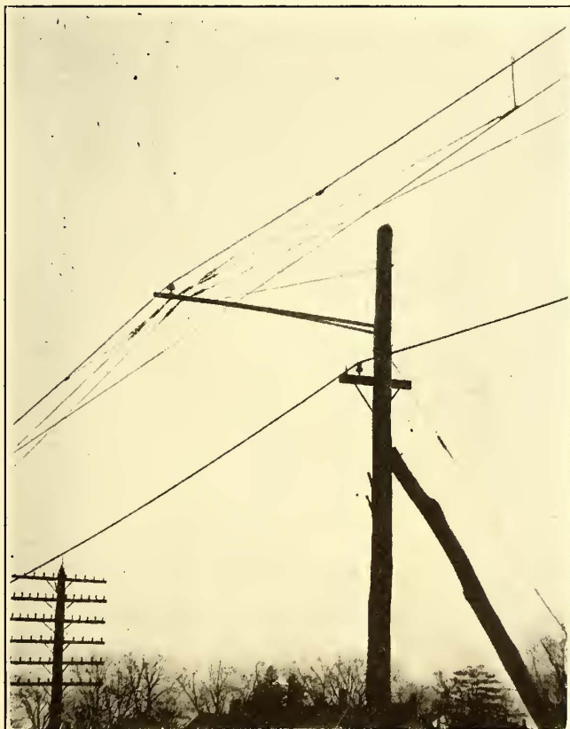
Catenary Lines After Test—Condition of Wires at Anchorage
