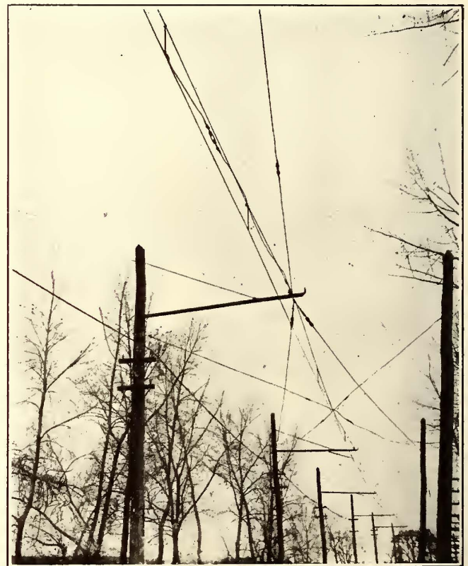
Catenary Lines After Test—Sagging Wires at Anchorage Approaching the Trolley Wire
