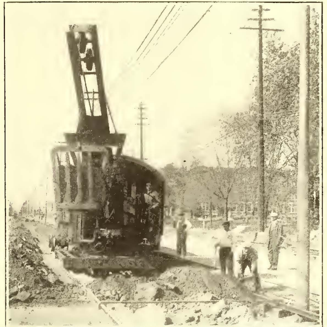
View of Shovel on Paved Street, Showing Cradle Support and Wide-Gage Track
