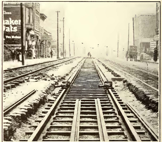
Romapac Rail—Ends of Head Rails Held by Jacks to Prevent Slipping During Crimping
