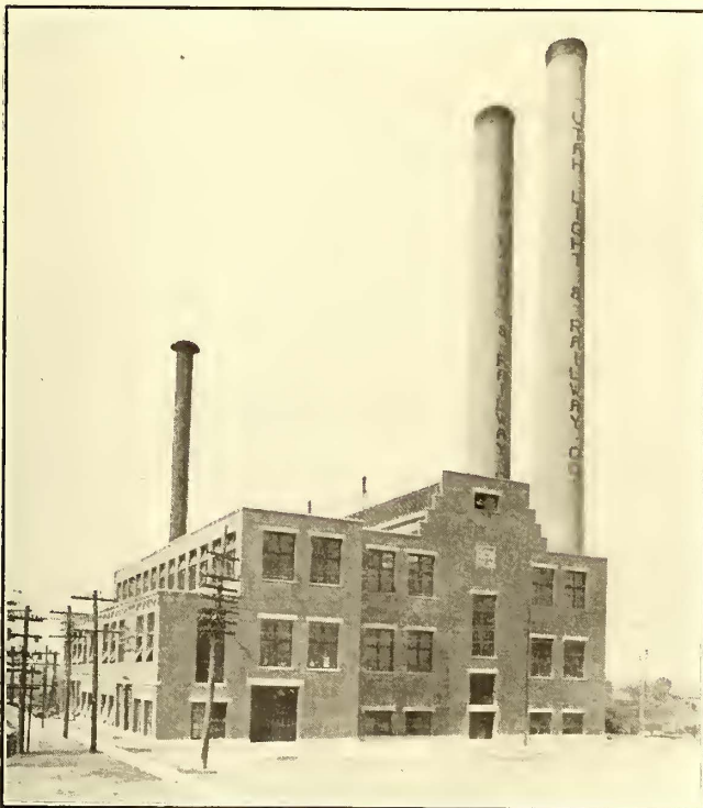
Utah Light & Power—General View of Salt Lake City Power Plant
