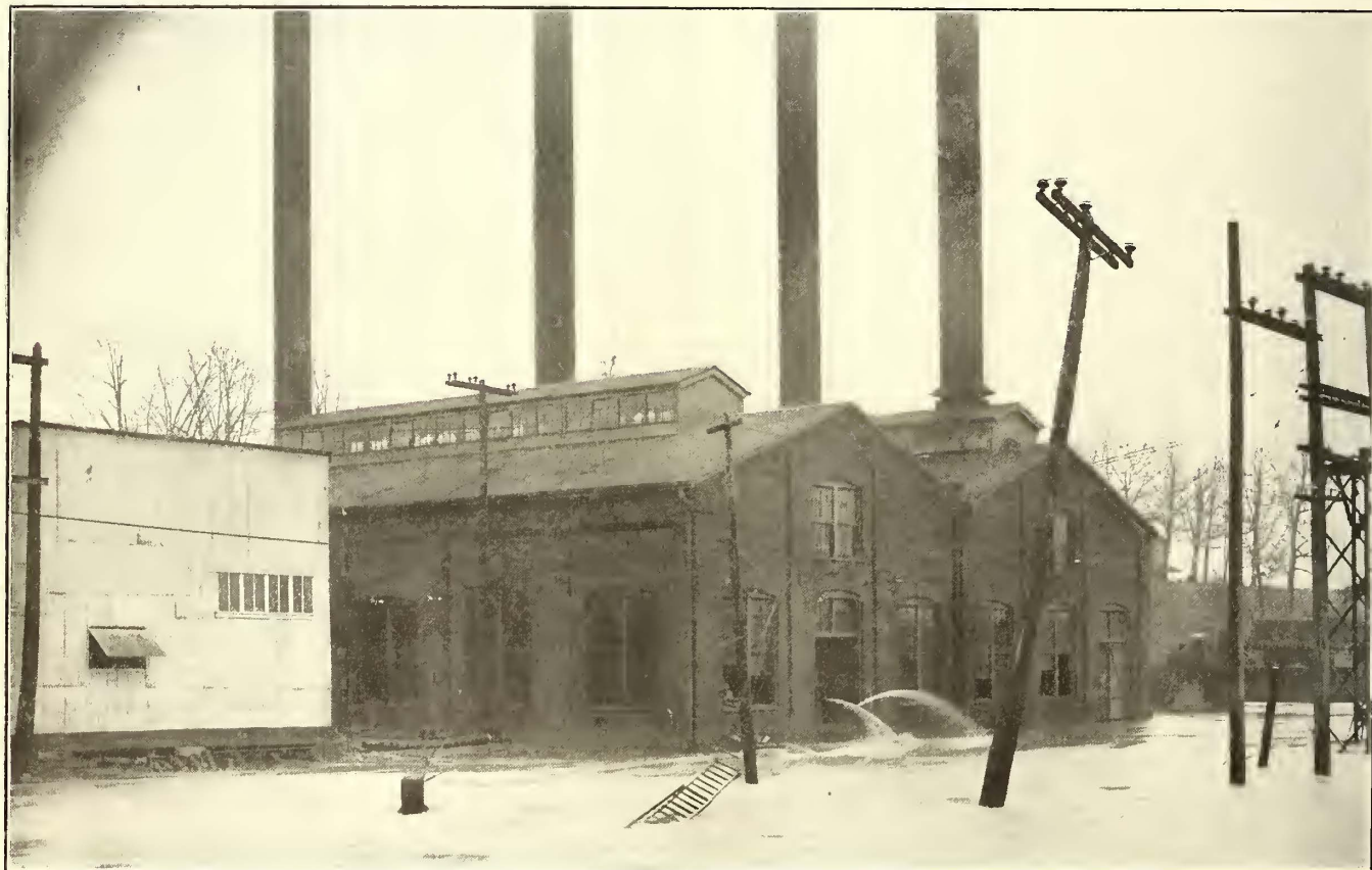
Flood Disaster—Power Station of Marion Light & Heating Company After Water Had Receded Two Feet
