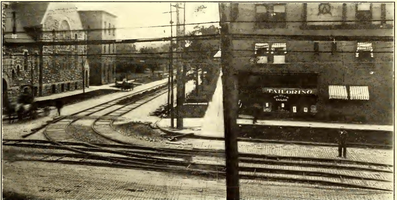
Cleveland Track—Temporary Track Laid on Surface of Pavement to Permit Routing Cars Around a Closed Section of Street
