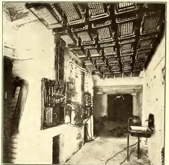
Third Avenue Welding—Resistances and Control Apparatus in Basement
