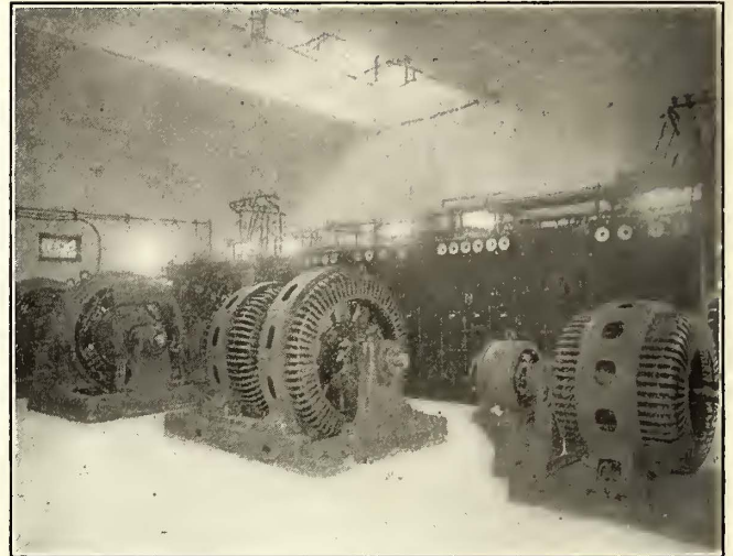
C., P. & E. Power—Interior View of Willoughby Substation, Showing Rotary Converters and Frequency Changers
