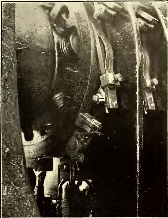
Collector Rings of Richmond Rotary Converter
