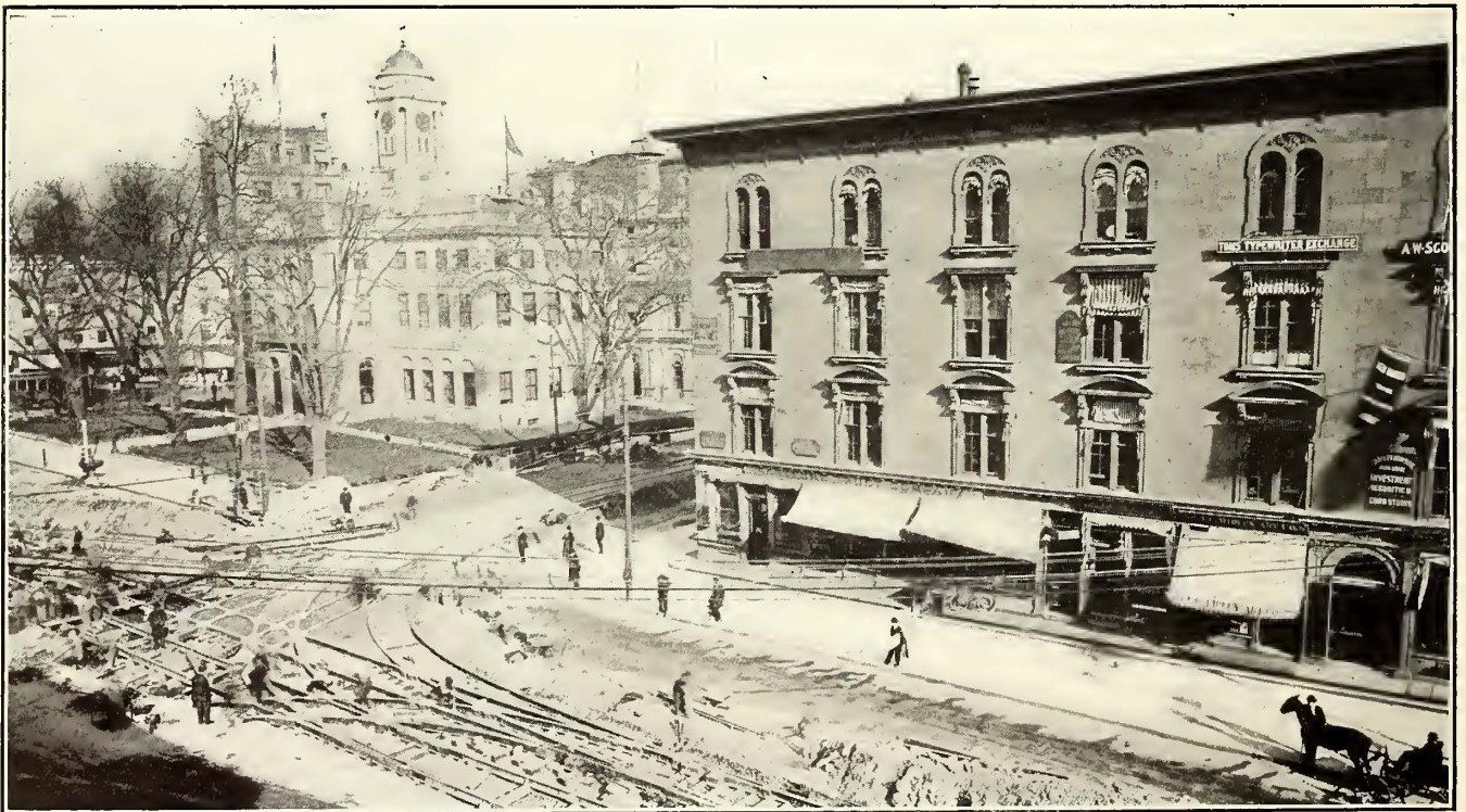
Connecticut Way—Special Work with Special Steel Center Construction Being Installed at the Corner of Pearl and Main Streets as Part of Loop Around Hartford City Hall
