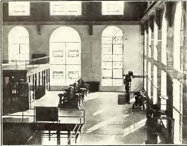
Northern Ohio Power—View of West End of Turbine Room Showing Engineer's Office and Local Substation
