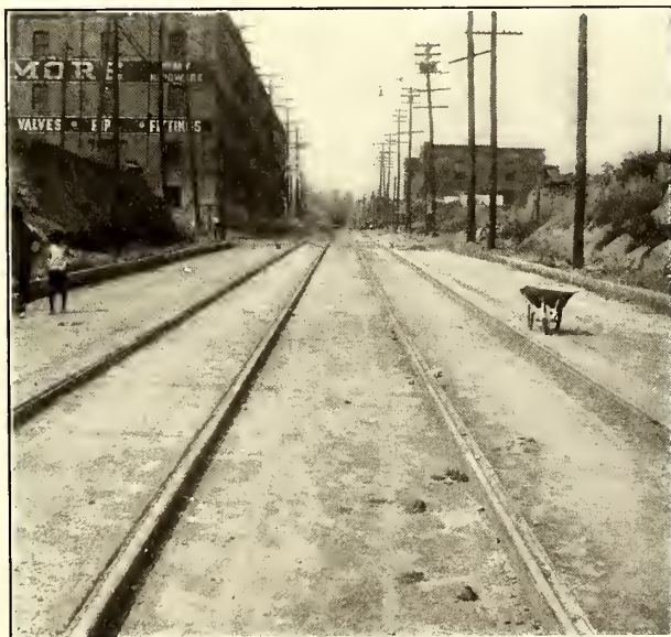
Girder-Rail Track with Tie Rods Covered Ready for Paving, Memphis Street Railway
