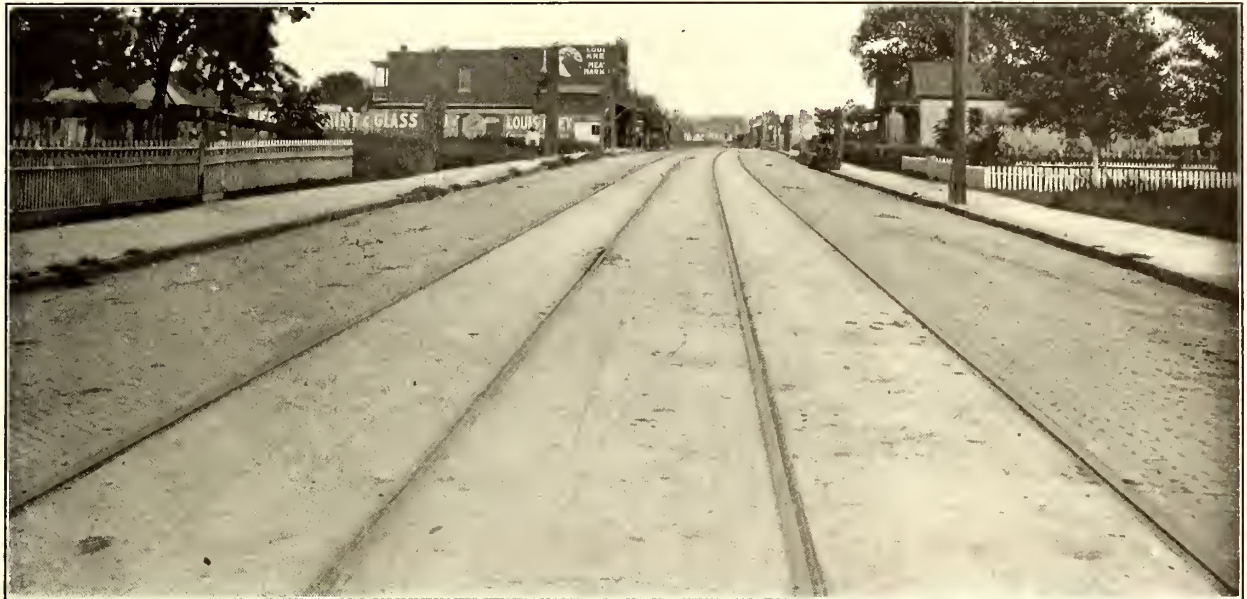
T-Rail with Paving Protector in Concrete Paving After Five Years' Service, Memphis Street Railway
