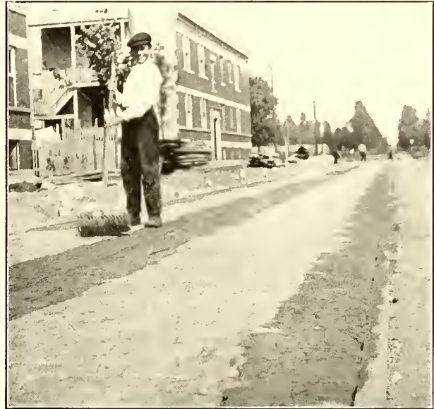
Grouted Paving Along Rails with Space Between Ready for Asphalt Filling, Chicago City Railway
