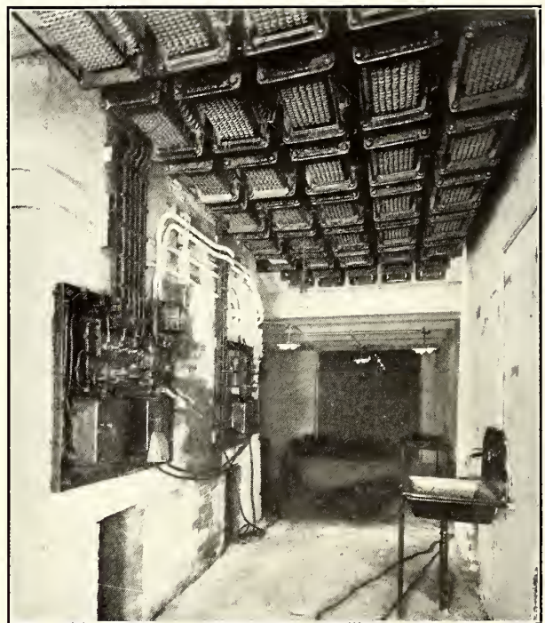
Old Grid Resistance for Reducing Line Voltage for Electric Arc Welding, Third Avenue Railway, New York
