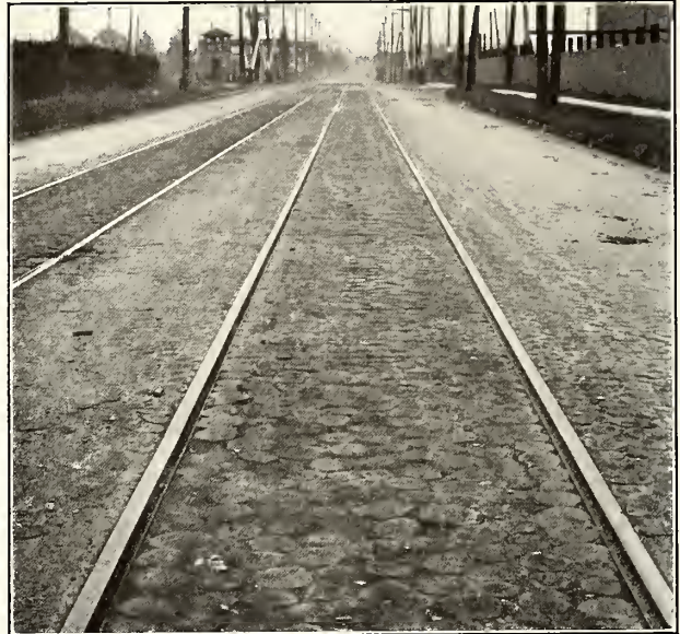
Detroit United Railway—Result of Modern Maintenance of Rail Joints by Lifting and Grinding
