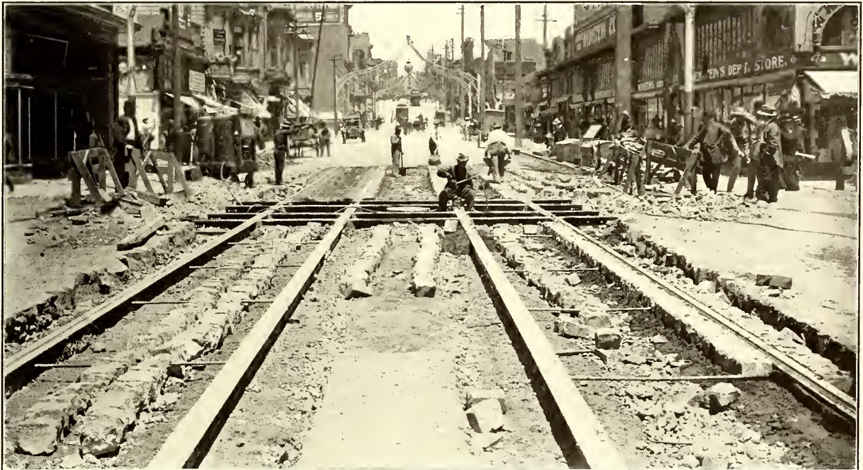
Laying Granite Block Paving on Mortar Bed, United Railroads of San Francisco
