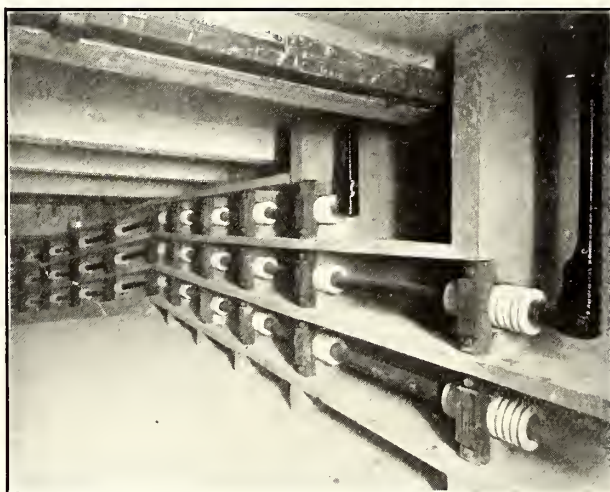
Generator Leads in Cable Vault, Northwest Station, Chicago
