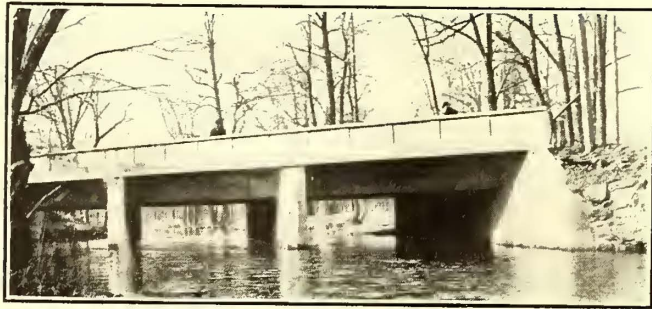
Connecticut Way—Concrete Girder and Slab-Paneled Side Bridge Which Replaced Pratt Truss and Trestle Structure Between New Haven and Cheshire
