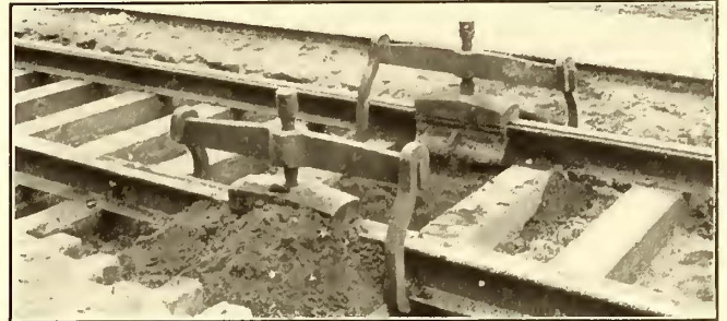
Brooklyn Joints and Ties—The Mold Complete and Ready for Pouring; Inverted C Clamps Used
