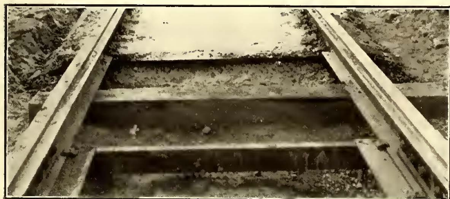
Brooklyn Joints and Ties—Detail Showing Wedge Tie Clips Between Plates and Rail; Also Concrete Base for Paving
