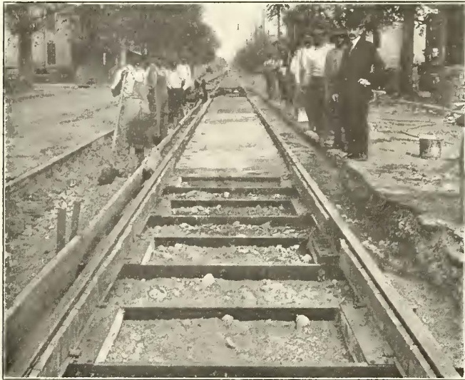
Dayton Installation, Where Ties Were Concreted at the Yard and Tamped to Line
