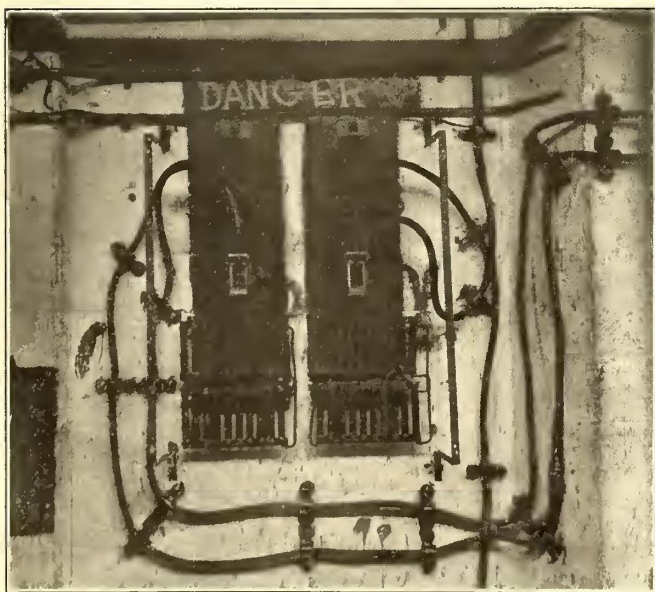
View of Contactors
