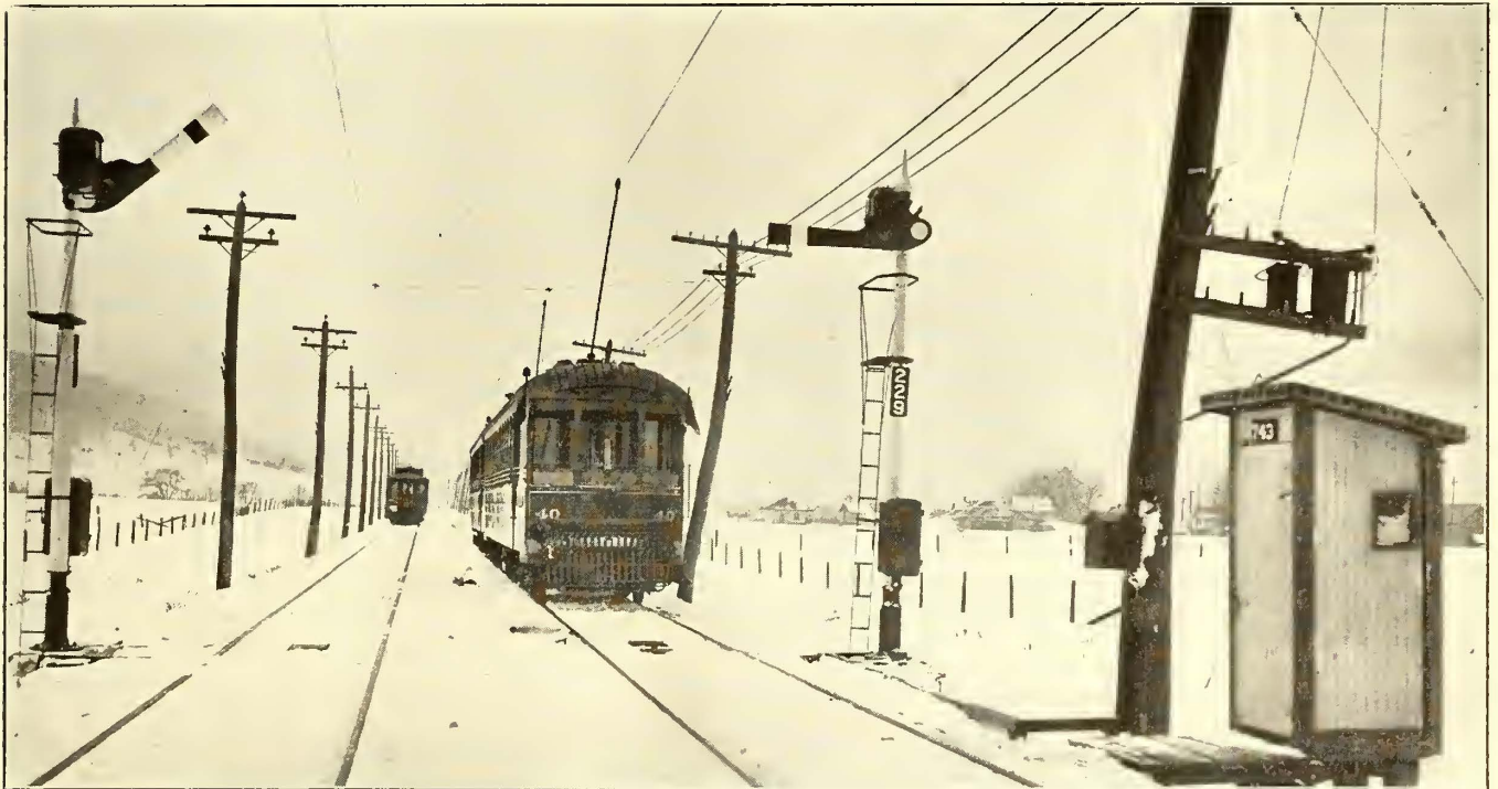
Utica Signals—East-Bound and West-Bound Signals and Telephone Booth Near Frankfort Substation
