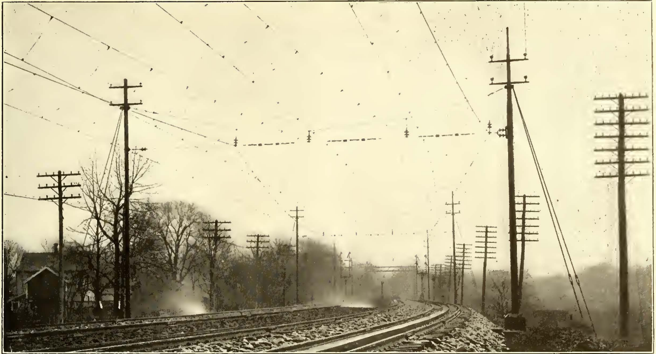
Philadelphia Electrification—Curve on Experimental Section Equipped with a Special Type of Flexible Hanger Supporting a Single Contact Wire
