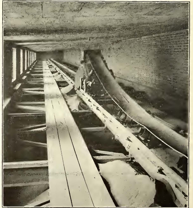
Philadelphia Rapid Transit Company—Belt Conveyor Distributing Sand in Carhouse
