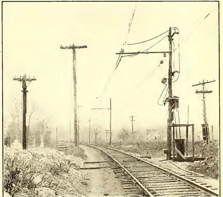
New Haven Electrification—Fig. 20—Track-Feeder Transformer on New Canaan Branch
