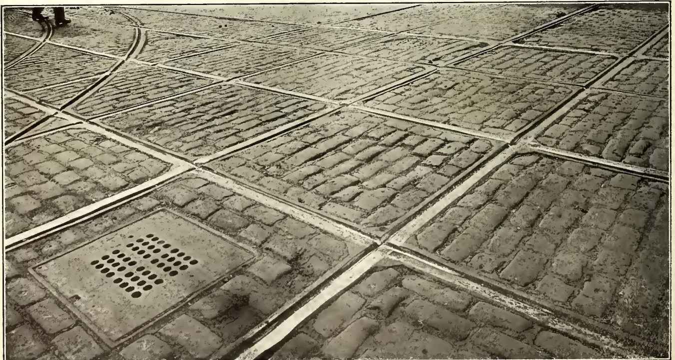
Chicago Special Work—Fig. 12—Showing Chipped Points and Cold Rolling in 90 Deg. Manganese Crossing, Installed February, 1911; Traffic, 345 Wheels Per Hour
