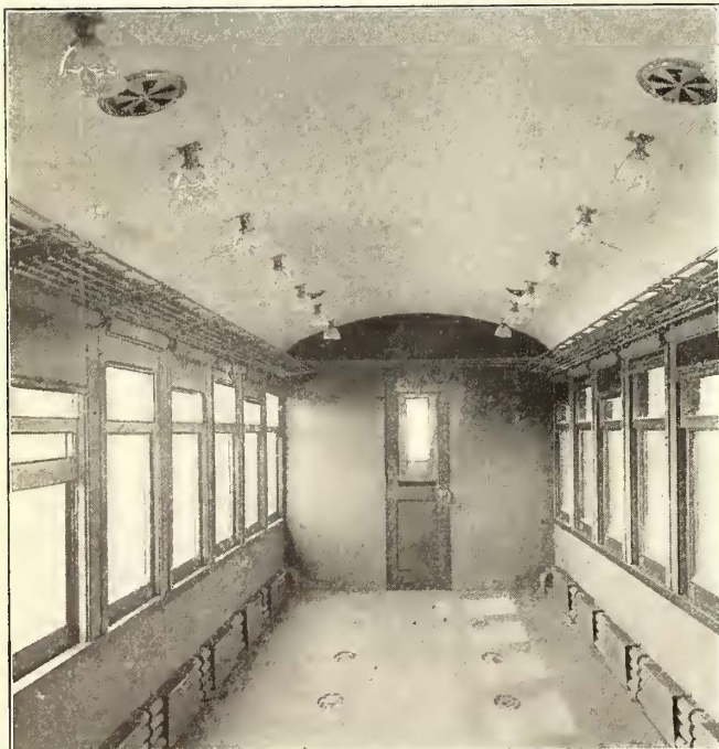
Michigan Cars—Interior of Passenger Compartment with Seats Removed, Showing Arrangements of Lights and Heating Coils
