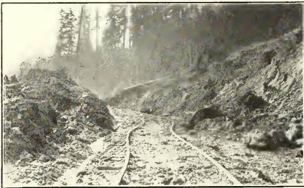
Seattle Municipal Railway—Example of Rehabilitation Work on Highland Park & Lake Burien Railway
