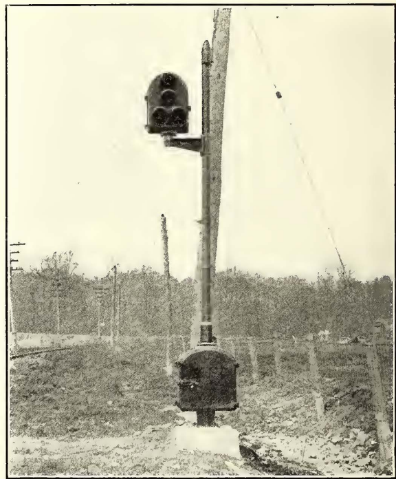
Signal of Trolley Contactor System as Mounted on an Individual Pole
