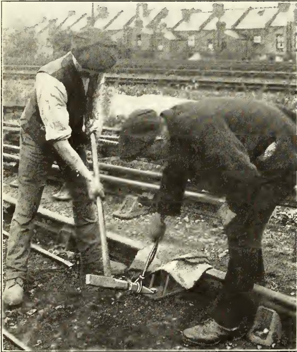
SAFETY FIRST—GREAT WESTERN RAILWAY—SAFE WAY BECAUSE THE BAGGING WILL CATCH THE BOLT HEAD
